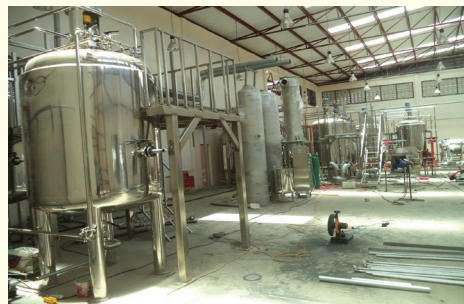
Installations in the production area at Soroti Fruit Factory the factory will be commissioned in 2018
